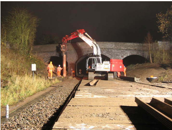
The Movax was tracked over on timber mats to protect rail lines
