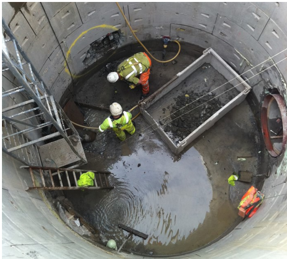
Members of the A E Yates Team Working at the base of the Shaft
